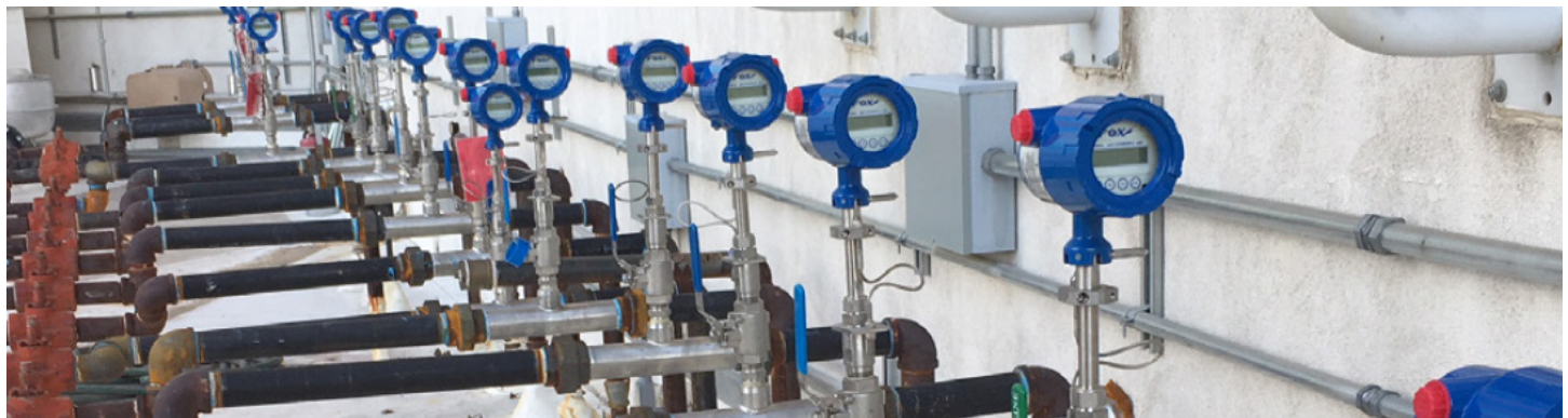
FT1 meters installed for natural gas sub-metering at a major hotel/casino in Las Vegas, NV.
