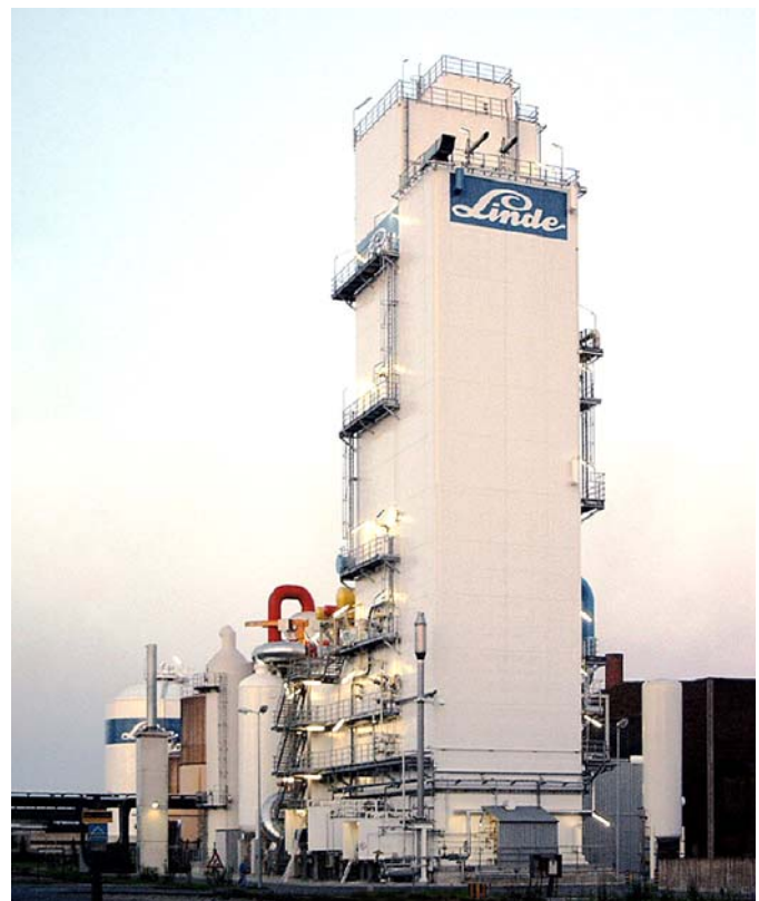
Air separation unit
